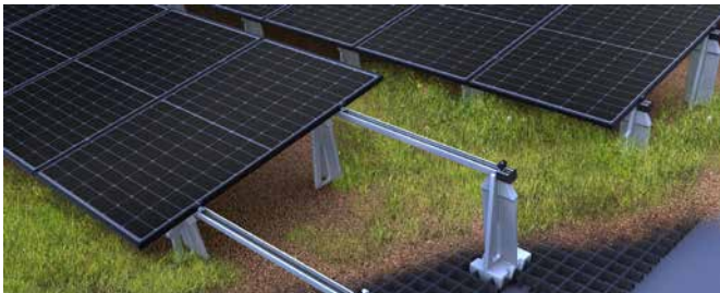
Green roof system south*
